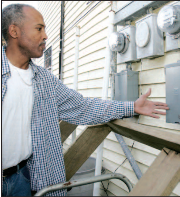
Walter Vine, an experienced contractor, used his knowledge to cut through the red tape to get power to his home and others on his street who have returned home. Vine said his uncle a licensed electrician certified the work.
